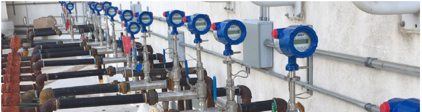
FT1 meters installed for natural gas sub-metering at a major hotel/casino in Las Vegas, NV.
